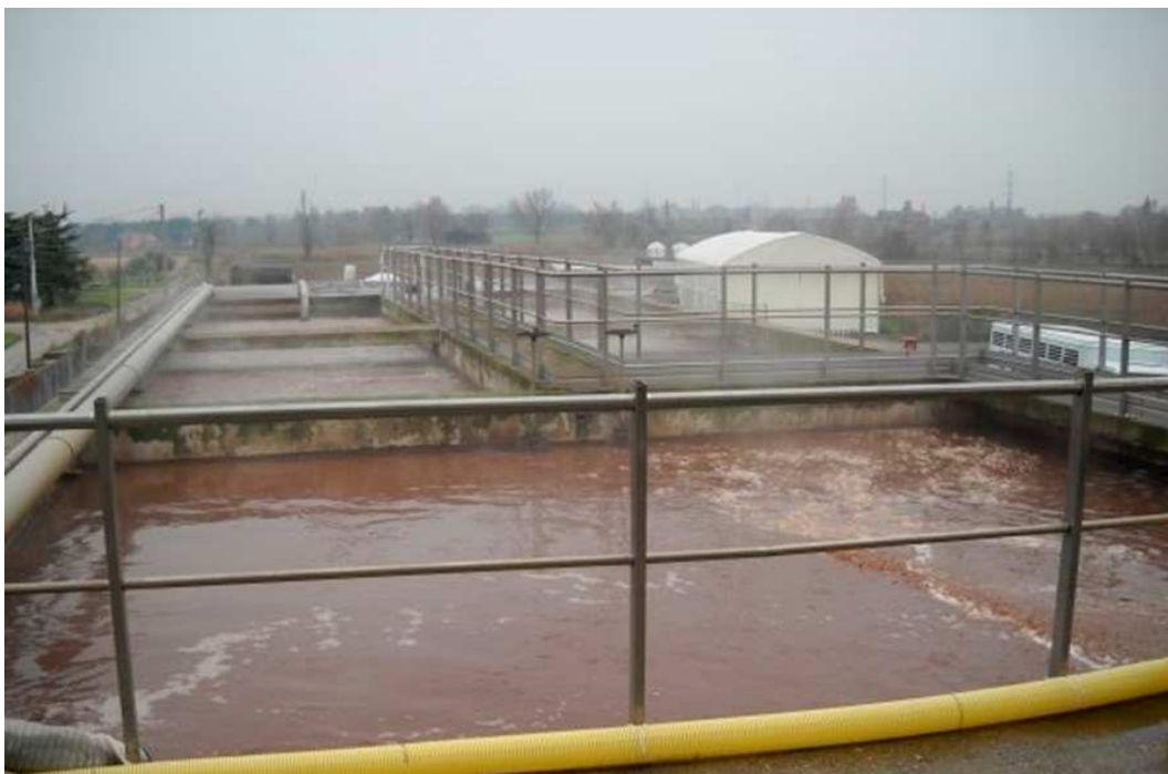
Figure 12.2: Photo of slaughterhouse wastewater treatment facility.
